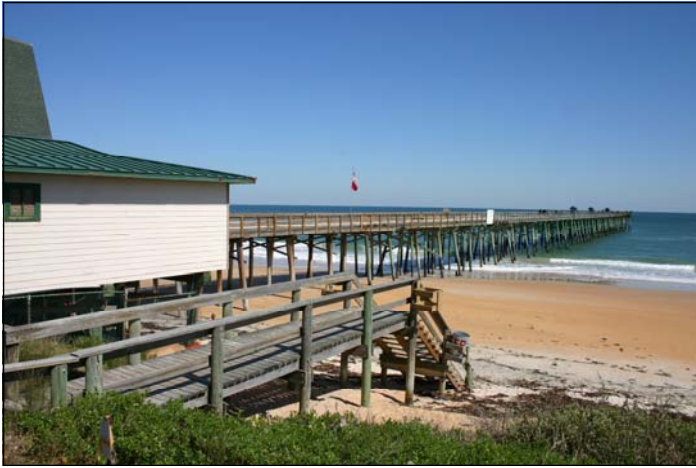
The Flagler Beach Pier re-opened on Friday August 7th to the delight of anglers and sightseers alike. The pier had undergone repairs to fix missing pilings and support beams.
